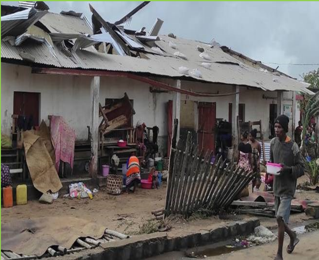
A man walks past a cyclone damaged building in Madagascar's Mananjary district.
